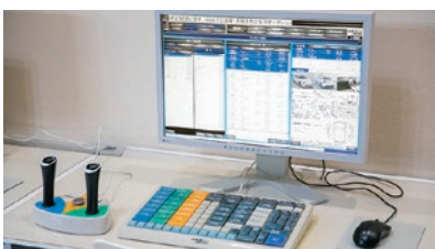
Dedicated satellite TV terminal
